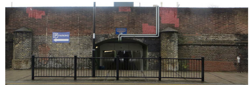
Perry Vale: inconvenient stepped access to the underpass
